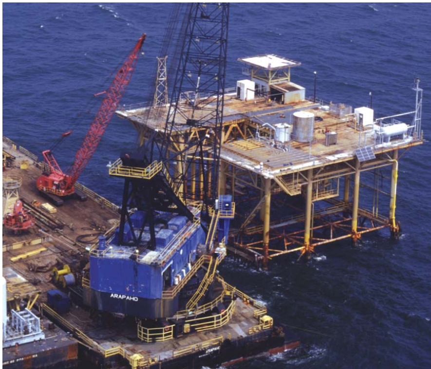
Figure 2. The Arapaho derrick barge performs a decommissioning operation in the Gulf of Mexico.
