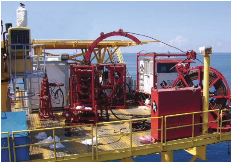
Deck space allows setup of coiled tubing unit in preparation for pumping operation.
